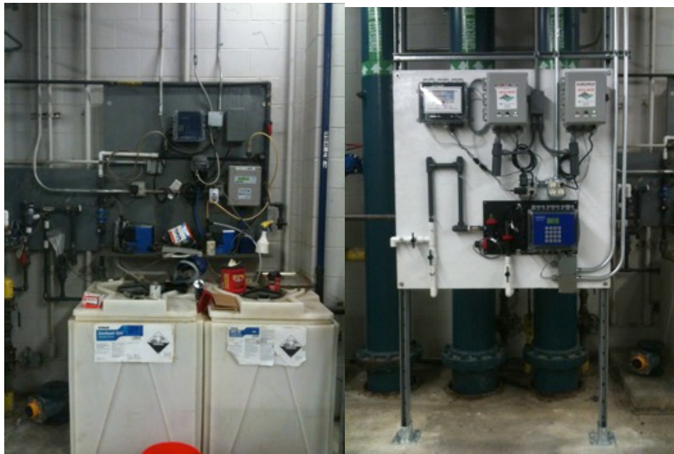
Above: Chemical treatment equipment (left) replaced by Zeta Rod system panel (right)
