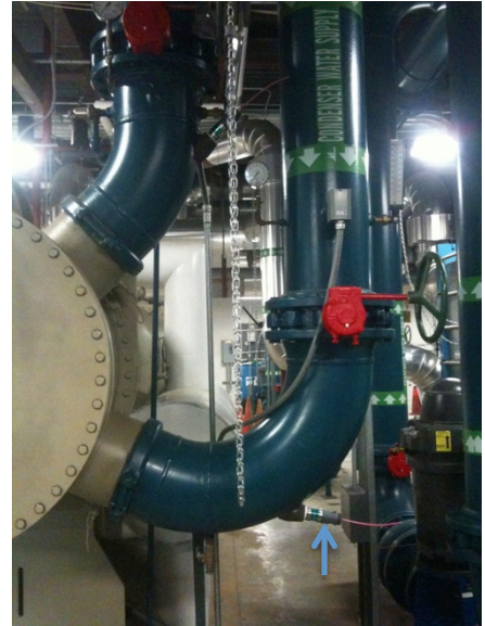
The picture above illustrates a typical insertion point of the Zeta Rod into the piping of each condenser water supply and return line for one of the chillers in Plant H.
