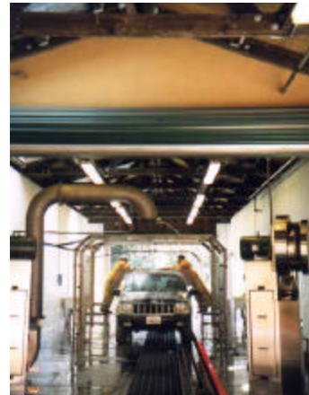
Installation of a Zeta Rod system eliminated tunnel odors and grime, and, by enabling use of the reclaim system, helped to significantly reduce per-vehicle wash costs.
